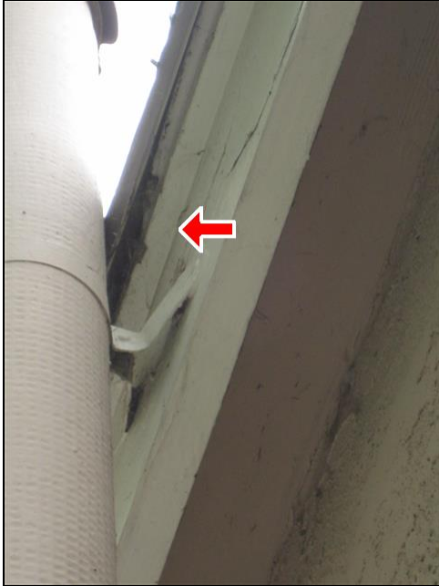
2.5 Item 1(Picture) Fascia damage
