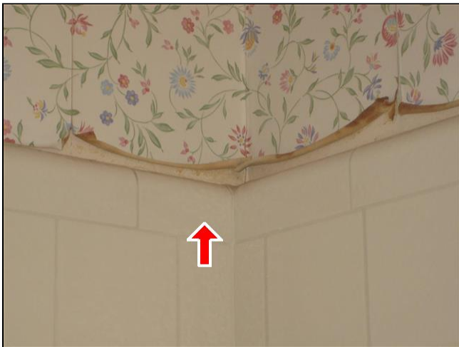
4.1 Item 3(Picture) Peeling wall paper
