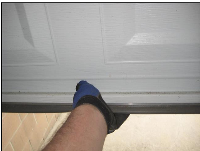
3.3 Item 1(Picture) Safety Issue
