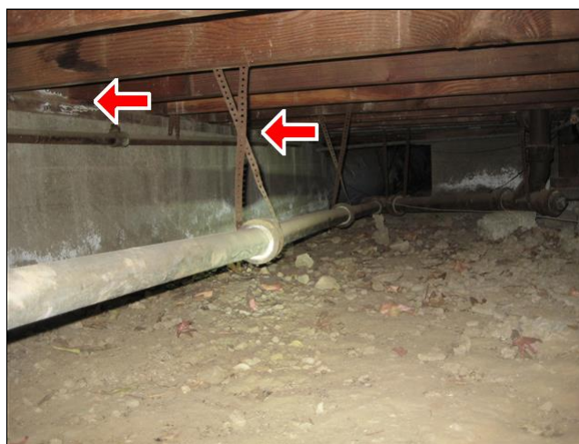
5.0 Item 4(Picture) No anchor bolts
