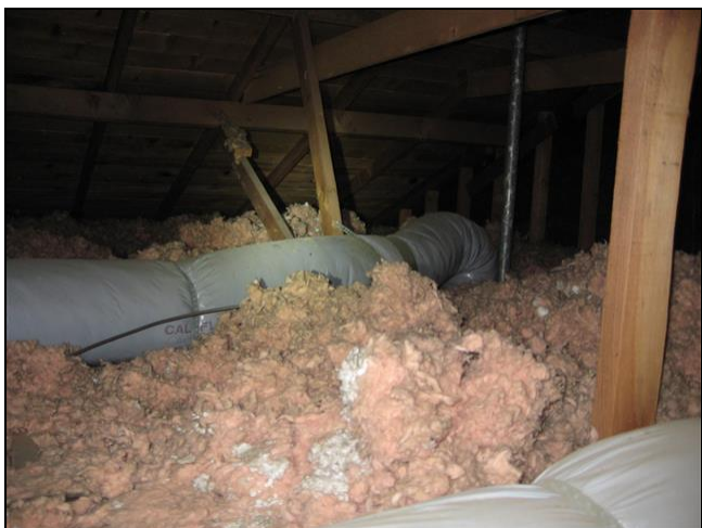
5.4 Item 1(Picture) Cannot see ceiling structure
