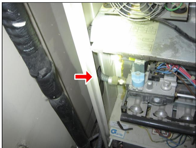
8.3 Item 1(Picture) Flexible gas line
