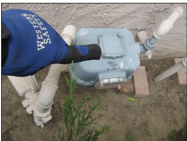
6.5 Item 1(Picture) Missing earthquake valve
