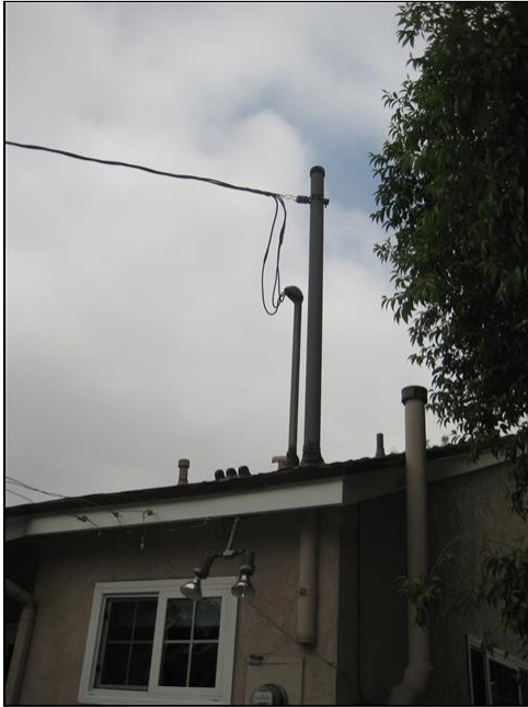
7.0 Item 1(Picture) Service entrance
