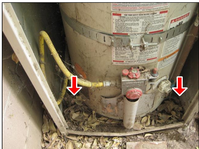
6.2 Item 3(Picture) Debris
