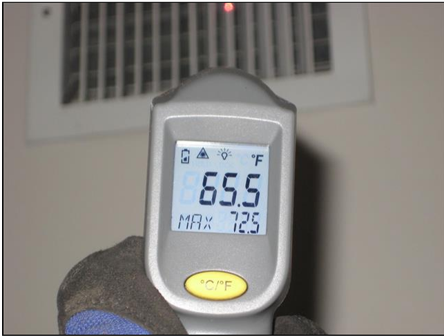
8.8 Item 1(Picture) Cooling
