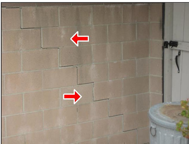
2.4 Item 3(Picture) cracks in leaning wall
