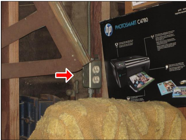
7.4 Item 3(Picture) Garage Outlets
