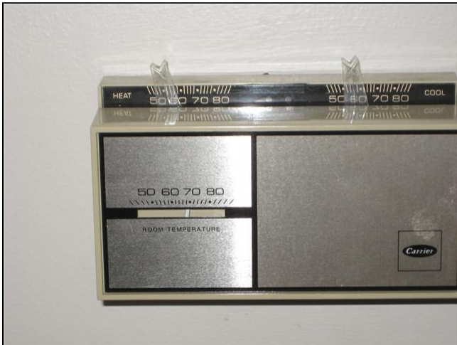
8.9 Item 1(Picture) Thermostat
