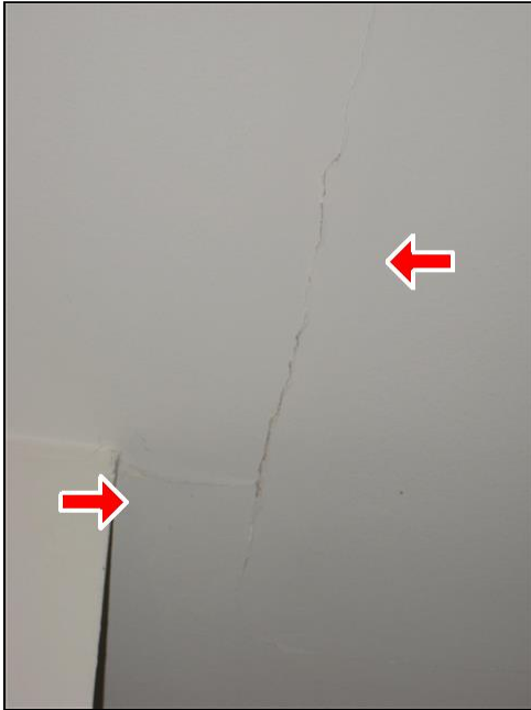
4.0 Item 2(Picture) Plaster damage
