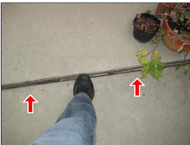
2.4 Item 5(Picture) Trip Hazard
