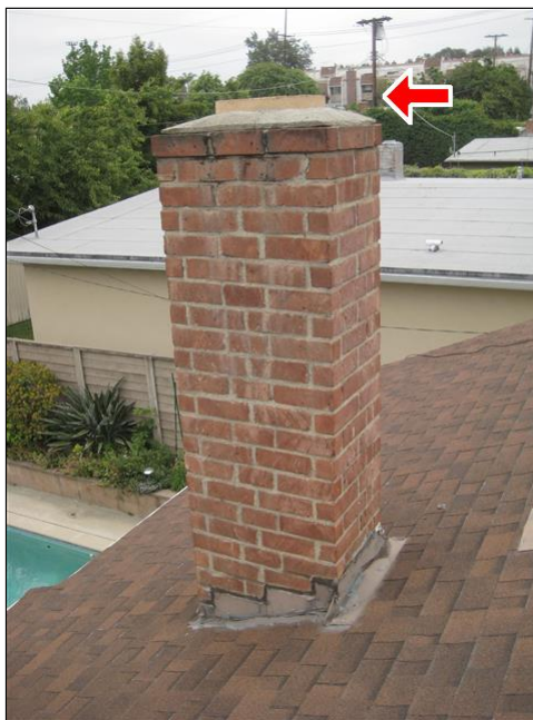
8.5 Item 2(Picture) Missing cap and arrestor
