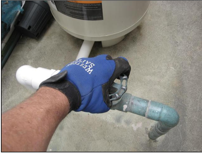
11.11 Item 1(Picture) Abandoned Pool fill valve
