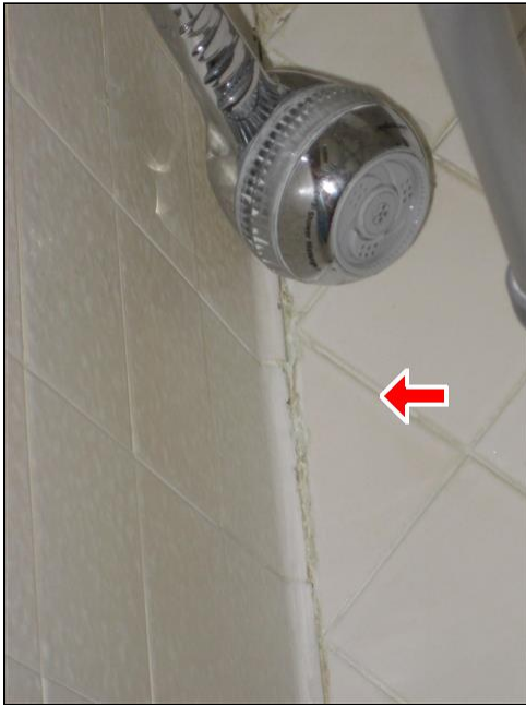
4.1 Item 5(Picture) Grout needed
