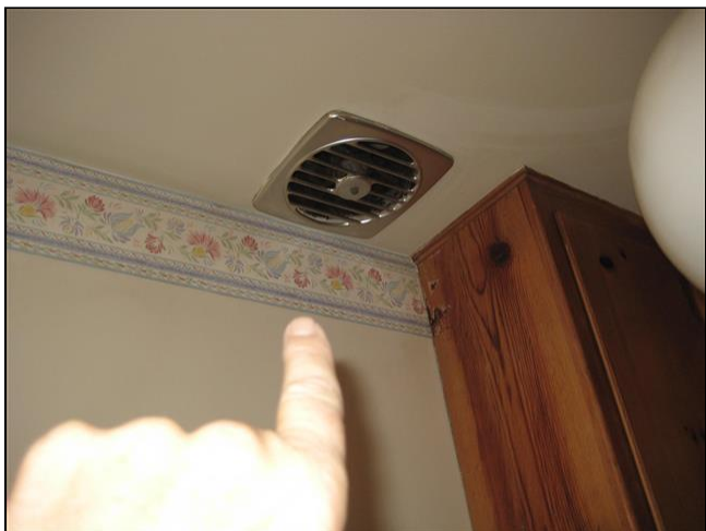
10.2 Item 1(Picture) Kitchen exhaust fan
