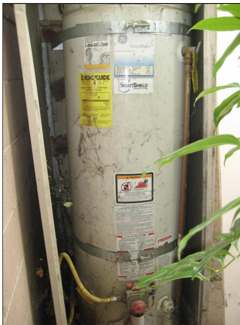
6.2 Item 2(Picture) Hot Water Heater
