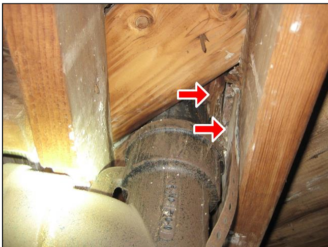
5.3 Item 1(Picture) Damage
