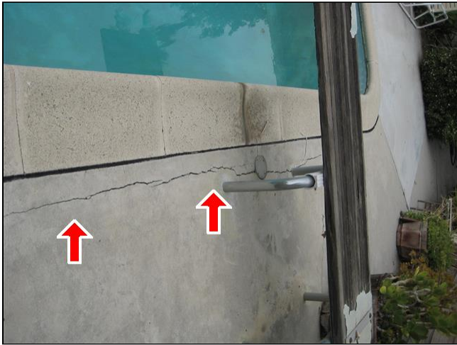
2.4 Item 7(Picture) Cracking at pool
