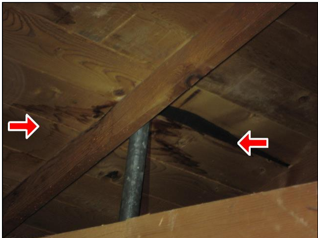
5.5 Item 3(Picture) wter stains
