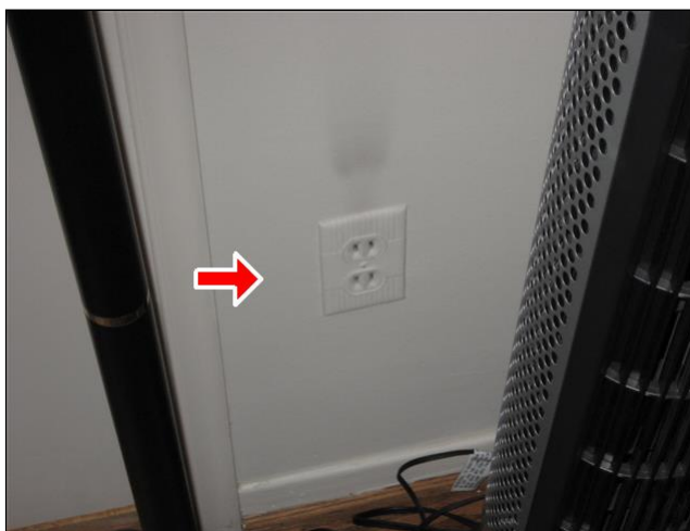
7.3 Item 4(Picture) non grounded outlet
