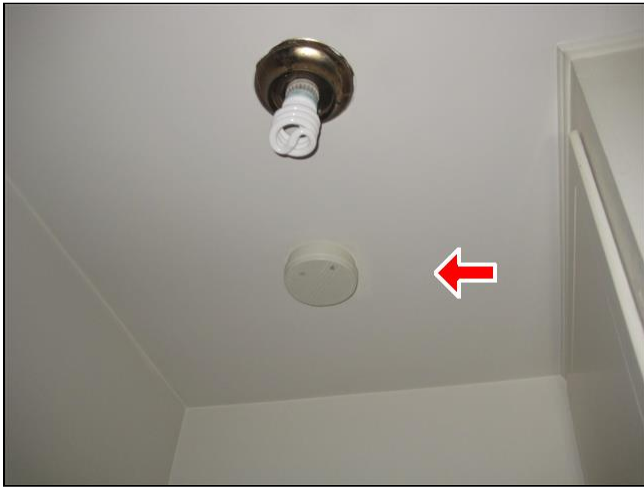
7.7 Item 1(Picture) smoke detector
