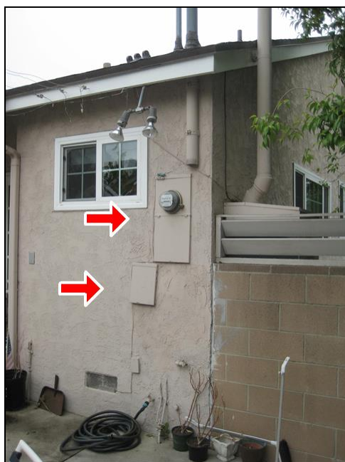
7.6 Item 1(Picture) Main Panel and sub panel
