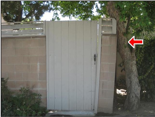
2.4 Item 1(Picture) Leaning wall
