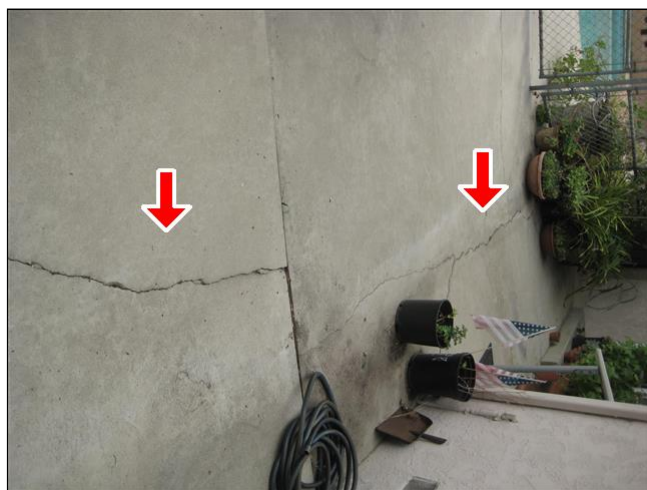
2.4 Item 6(Picture) severe cracking
