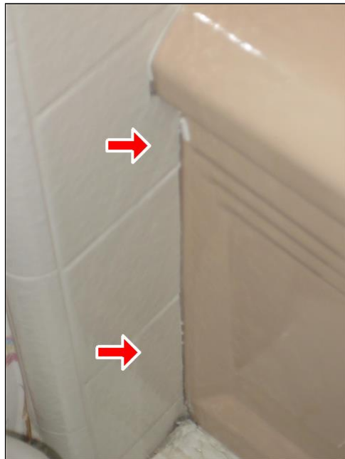
4.1 Item 4(Picture) Grout needed
