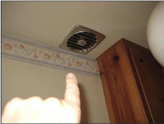
9.4 Item 1(Picture) Non working kitchen Exhaust
