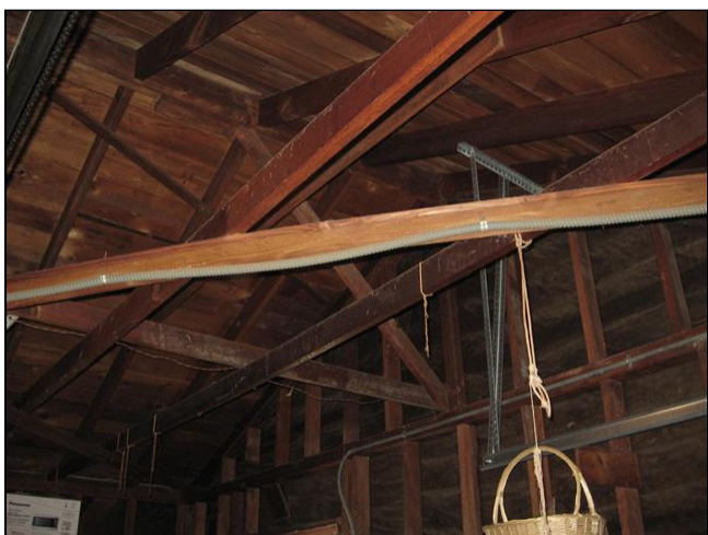
3.0 Item 1(Picture) Garage ceiling
