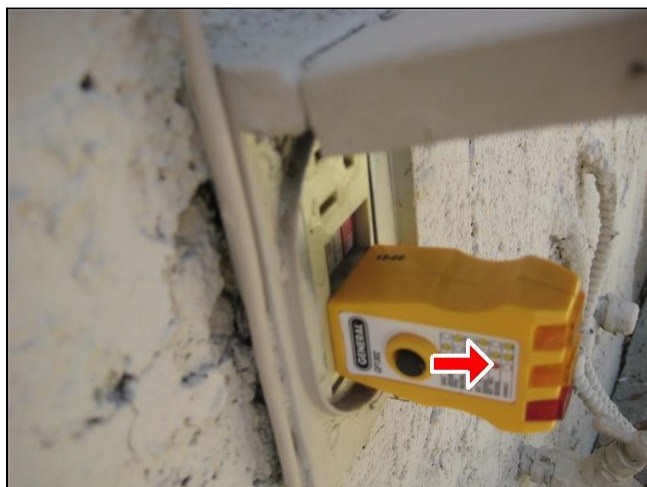
7.5 Item 1(Picture) GFCI no power
