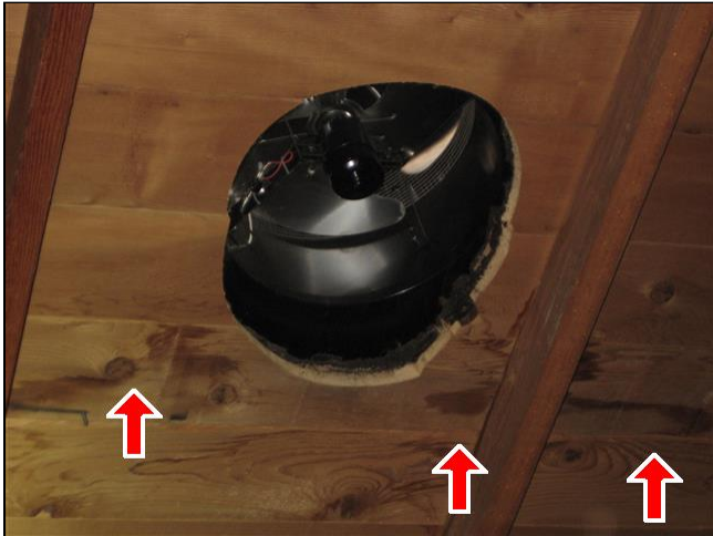
5.5 Item 2(Picture) Water stains
