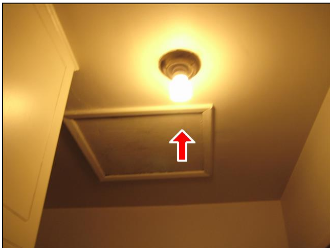
7.3 Item 1(Picture) Missing bulb cover
