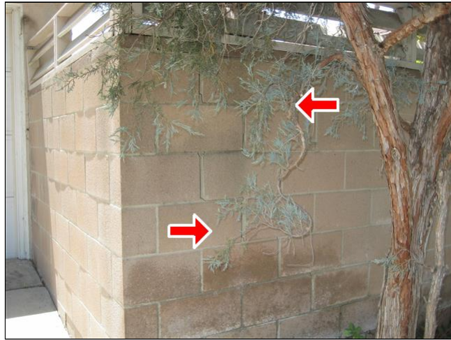
2.4 Item 2(Picture) Wall cracks
