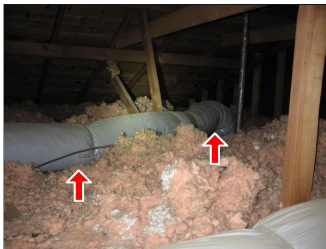
8.0 Item 2(Picture) Insulated ductwork
