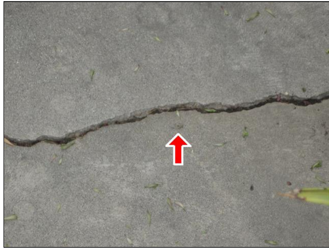
2.4 Item 8(Picture) Cracking near pool equipment and throughout
