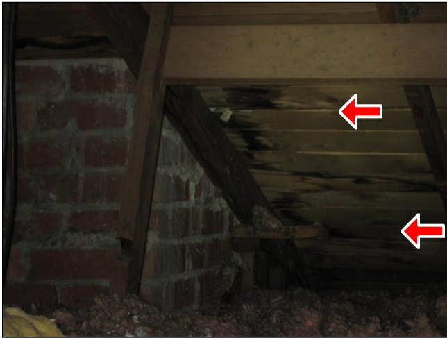
5.5 Item 1(Picture) Water penetration
